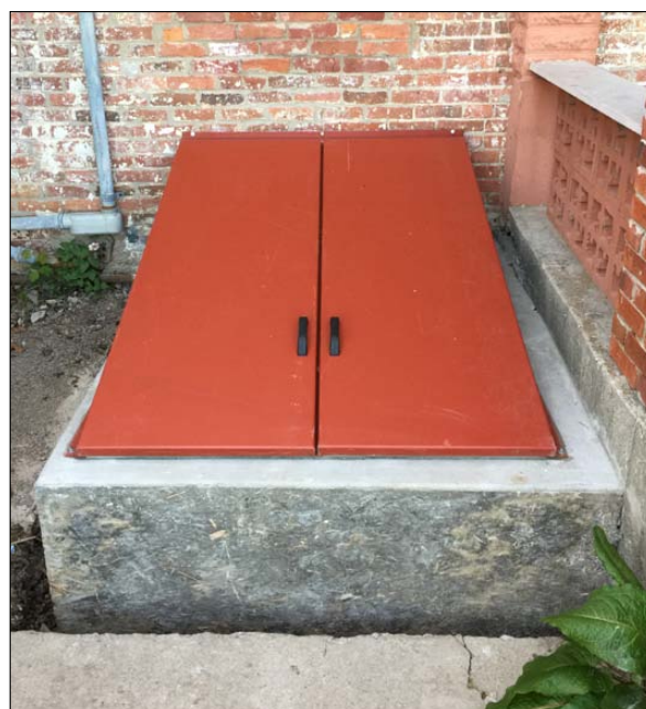
■ The new steel cellar doors were installed at the club Clean-up Day, May 14. The new doors should provide added security and should help eliminate water issues in the basement. The old steps/stairs were removed in order to put in the new concrete frame and the door, so those will need to be replaced.
