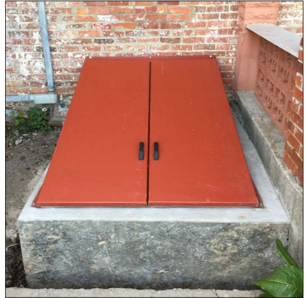
■ The new steel cellar doors were installed at the club Clean-up Day, May 14. The new doors should provide added security and should help eliminate water issues in the basement.
